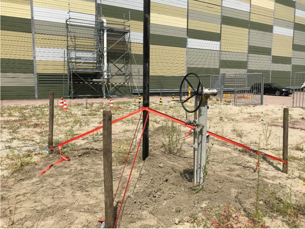
Figure 7. Vent stack DN100.
