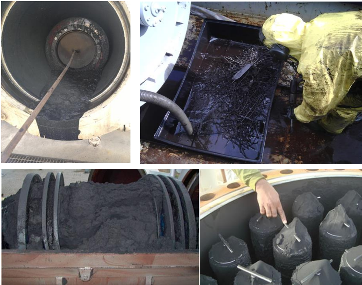
Figure 12. Examples of contaminants found in existing natural gas pipelines.
