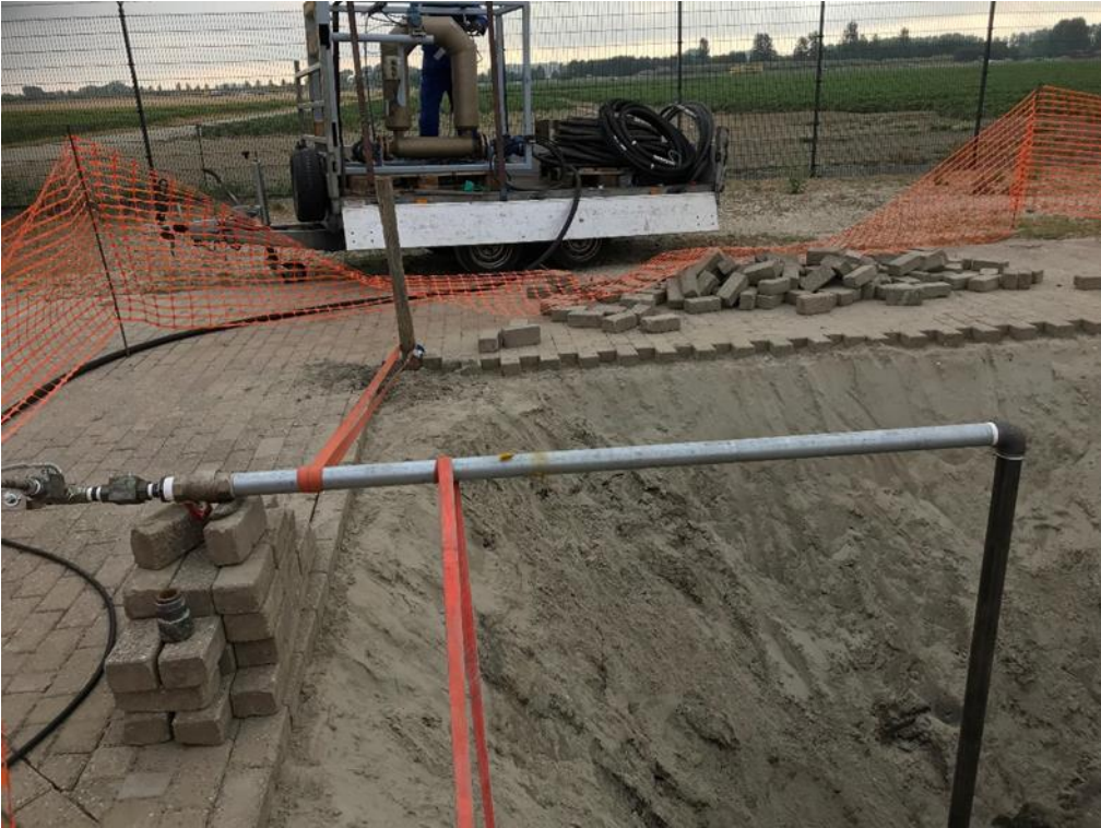
Figure 6. Nitrogen injection DN50, Coriolis flowmeter on the background.
